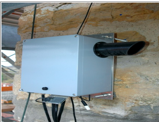
Pic 1: Dimetix Sensor installed at the historic building "Blauer Turm" in Germany.
